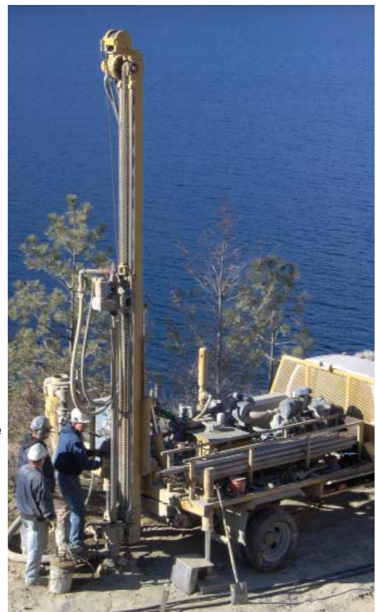
A team of technicians getting ready to drill holes for a vertical geothermal energy system
